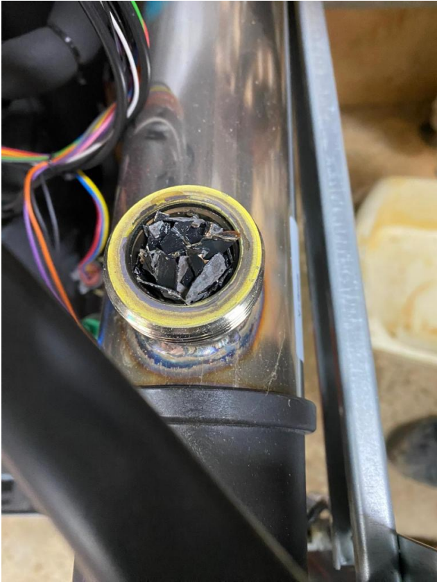
Corroded particles in the back up heat exchanger inside the heat pump
