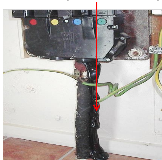
Cut-out with signs of bitumen leaking
