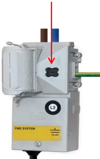
Earth terminal cover in place
