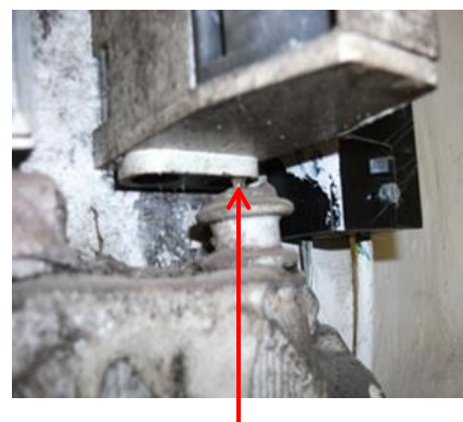
Visible bare conductors
