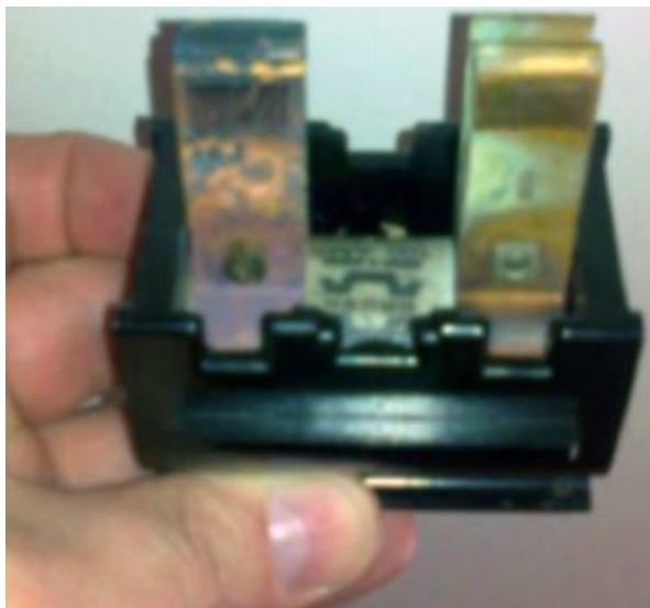
Weakened fuse carrier contacts
